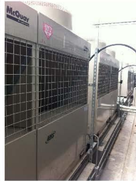
VRV MVAC systems for podium
