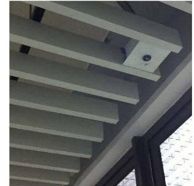
Daylight Dependent Lighting Control
