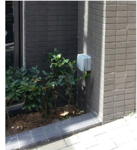
Charging Points for Electric Vehicles
