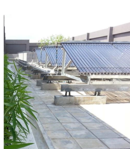
Solar Hot Water Panel
